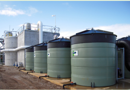
Busselton Wastewater Treatment Plant, WA
